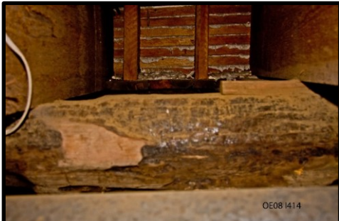
A close-up of a charred wooden beam
